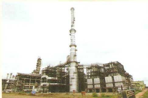
Mechanical works for HCU DHDT heaters for Bharat Oman Refinery, Bina, M.P.
